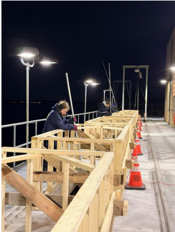
PWD staff working 12-hour shifts to clear ice from raw water intakes.
