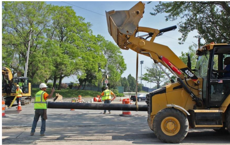
PWD crews replace a water main to ensure that the city's 3,000-mile network of water mains provides reliable delivery of safe, top-quality drinking water.
