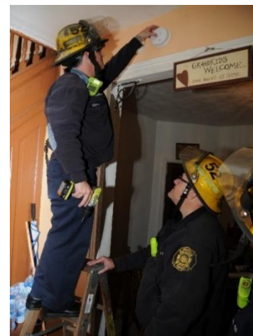
PFD members install a smoke alarm in a private residence. Donations and local contributions allow the PFD to provide these devices to households at no cost.
