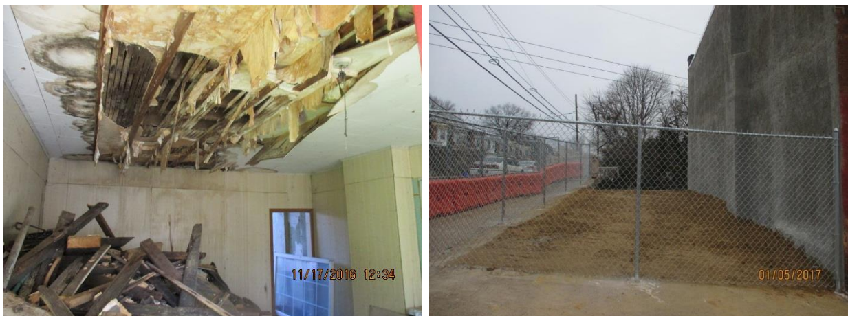
Before and after photos of a demolition on an imminently dangerous property that was directly adjacent to a SEPTA regional rail line.
