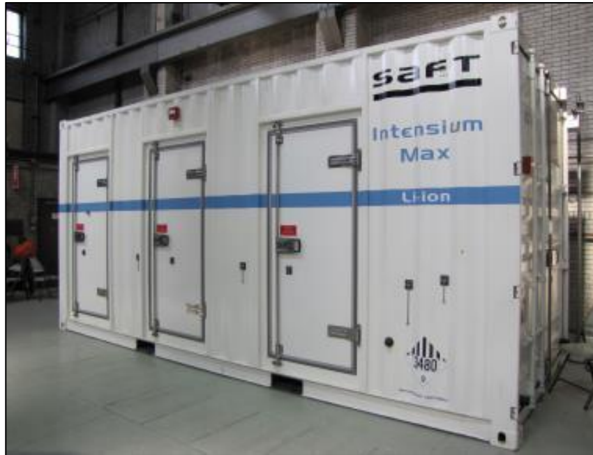
LITHIUM ION BATTERY AT LETTERLY SUBSTATION ON MARKET-FRANKFORD LINE
