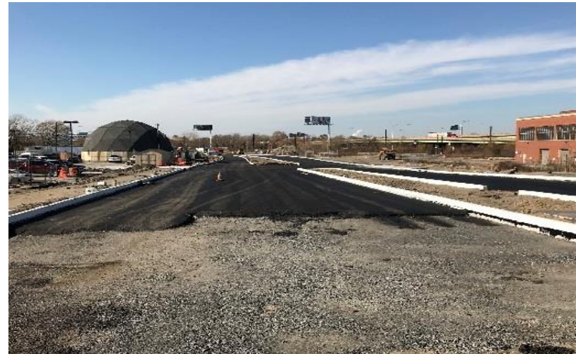
Reconstruction of Langley Avenue, part of ongoing access improvements to the Navy Yard. www.navyyard.org/
