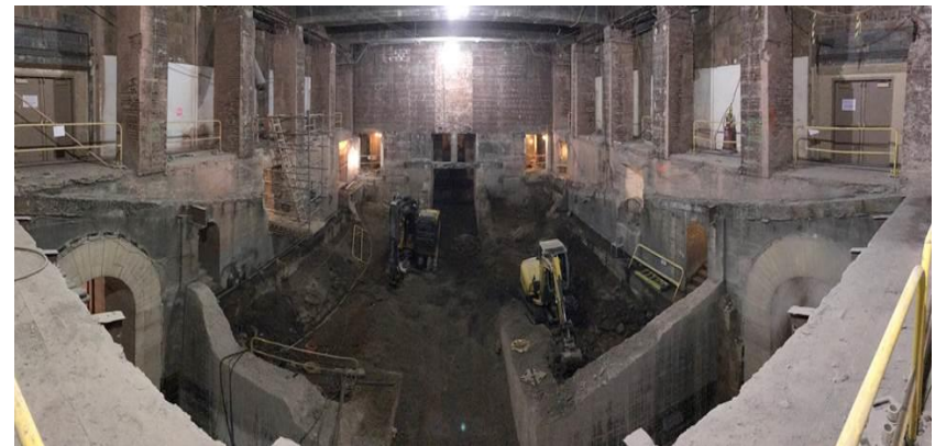
Space created within the heart of the Philadelphia Museum of Art by the demolition of the former Van Pelt Auditorium. A new public space called The Forum will be constructed here as part of the Core Project.
