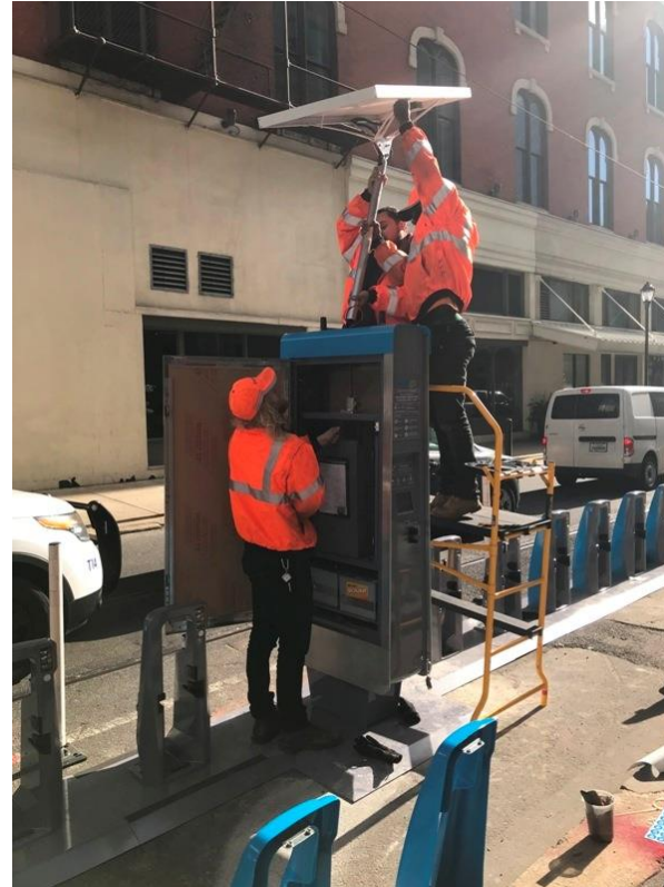
Installation of an Indego bike share station at 12 th and Walnut Streets
