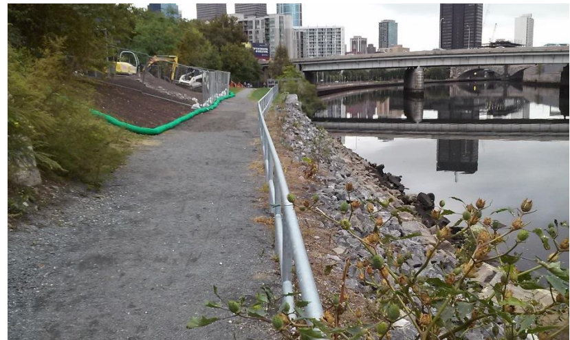
Reconstruction in 2017 of part of the Schuylkill River embankment and recreational path damaged by erosion in Center City
